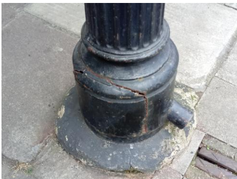
Example of fractured cast iron which required specialists to repair
