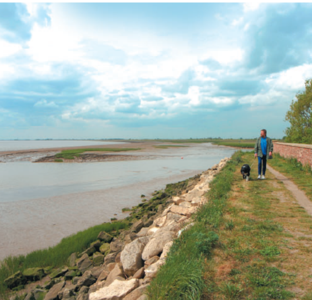
Flood defence at Brough
